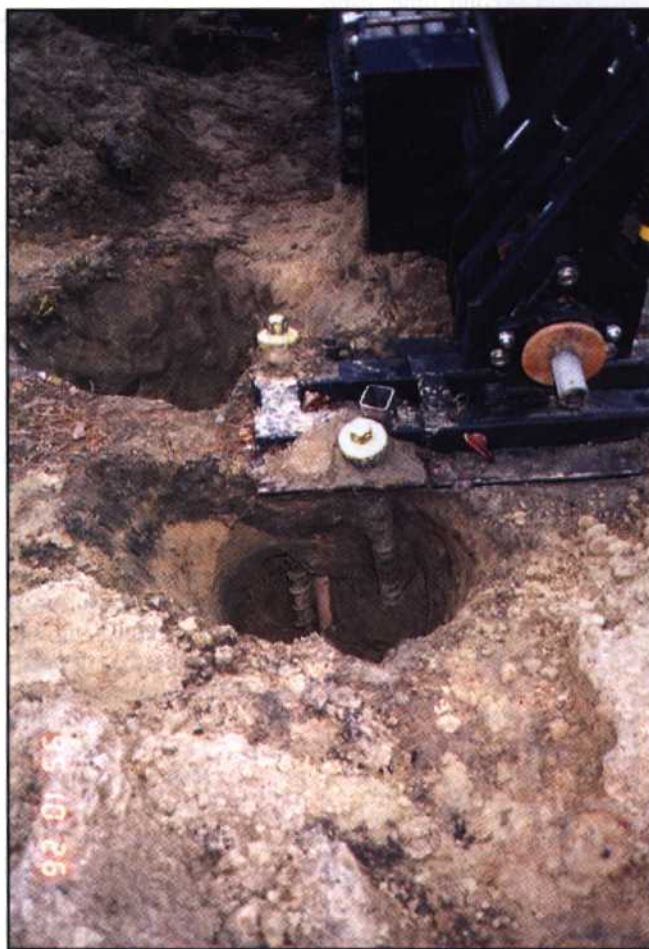
This drilling operator thought he only had to worry about gas mains across the street until he hit a 2-in. PE gas main. He even put three anchors within 4 in. of three gas lines, as this photo illustrates.
